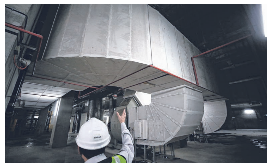
The mechanical ventilation system in the basement of the liquid treatment module of Changi WRP is used to keep the basement well-ventilated by drawing out air and pushing fresh air into the basement.
