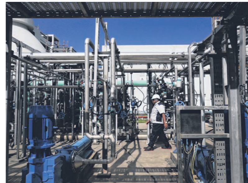
The thermal hydrolysis process facility helps to increase solids treatment capacity at the Jurong plant without the need to construct any additional digester. It also reduces digester footprint required for sludge management.
