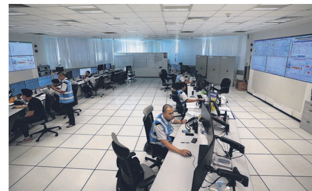
The main control room in the Changi plant is the heart of its operations. Here the operators can handle equipment remotely and monitor the treatment process of used water.
