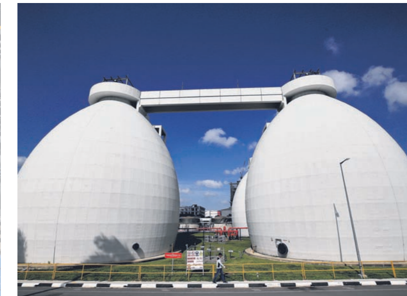
Sludge from the used water treatment process is converted to methane-rich biogas in egg-shaped digesters at the Jurong plant. This biogas, which serves as fuel in gas engines to generate electricity, is used for in-plant power generation.
