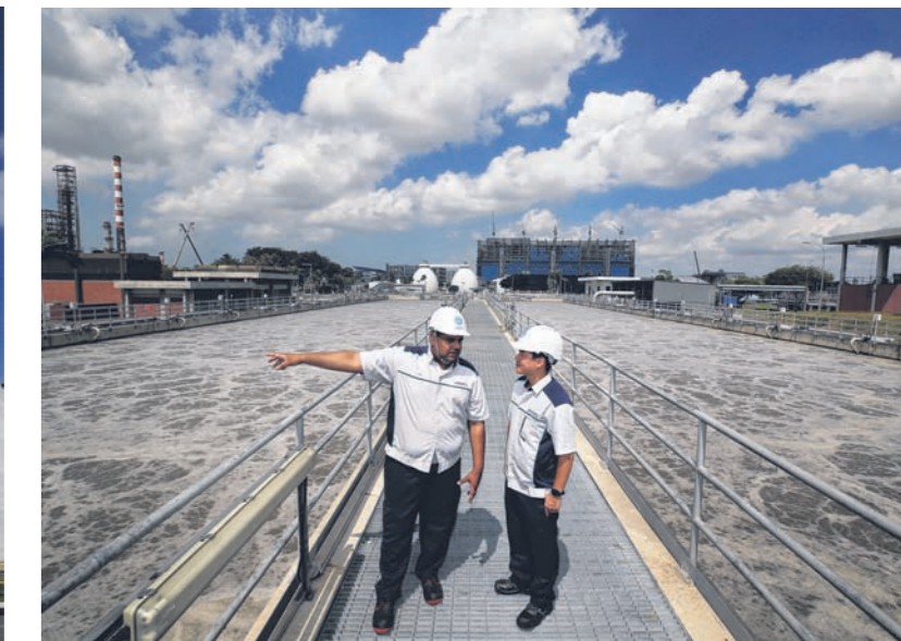
Senior engineer Balasubramaniam Jeyanathan (left) and engineer Lim Seng Leong observing the treatment process of industrial used water at the aeration unit of the Jurong plant.
